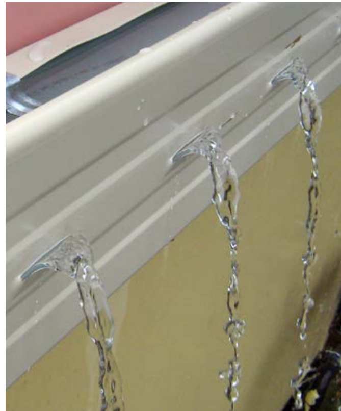
Typical overflow from slotted gutter.
