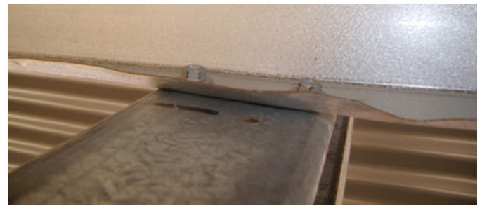
Poor support conditions (flange not sitting flat).
