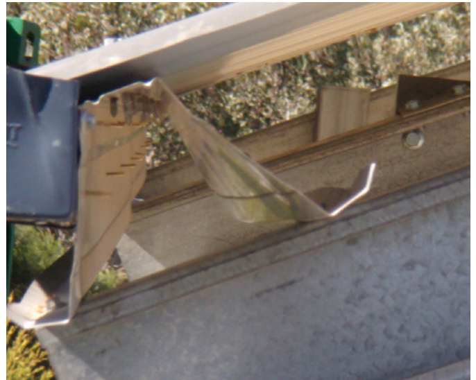
Spread of TOPSPAN® During Incorrect Installation.
